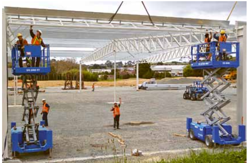
MS Engineering was on a tight timeline to fabricate and erect the structural steel work for the Mitre 10 Mega store, with just seven weeks from start to finish.
